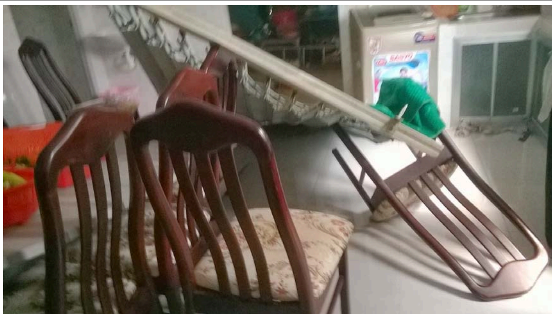
Picture 4: The metal back door of Nguyen Bac Truyen house was destroyed on Feb 9, 2014
