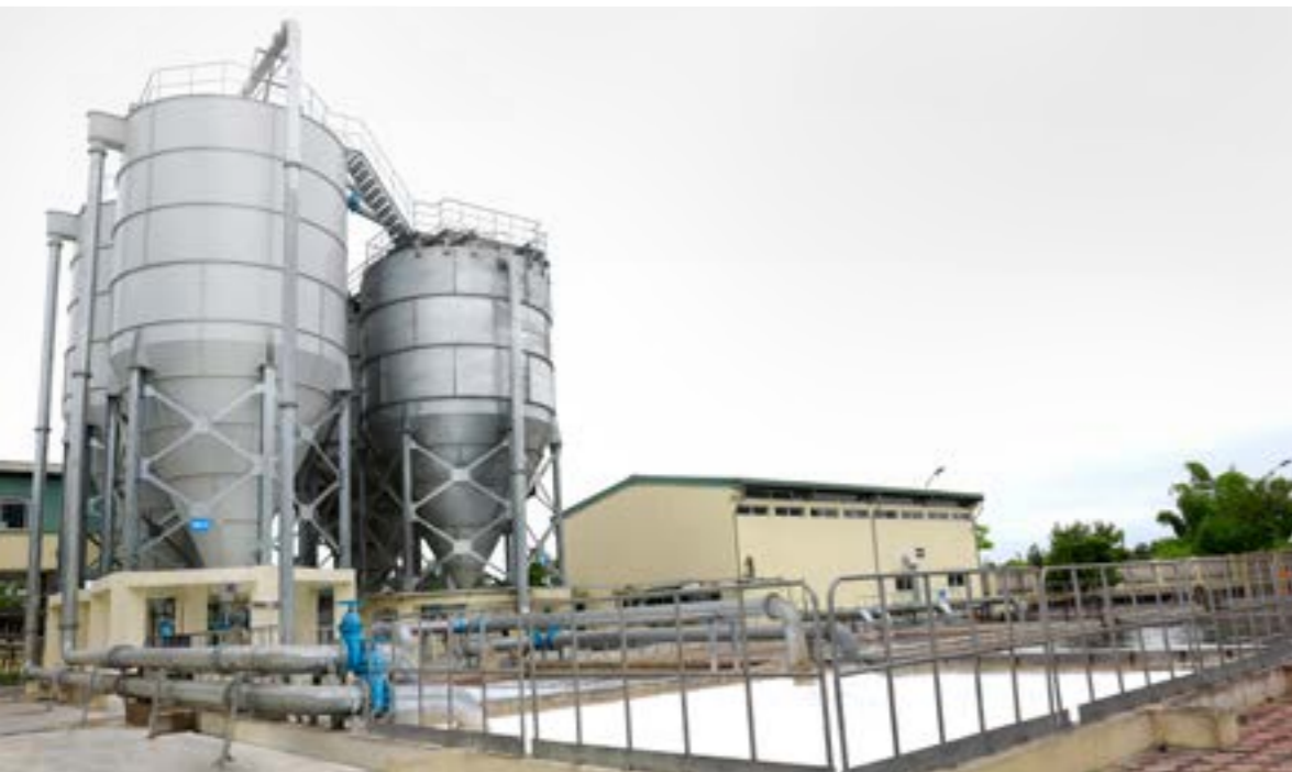
Vicostone's water circulating silo system
